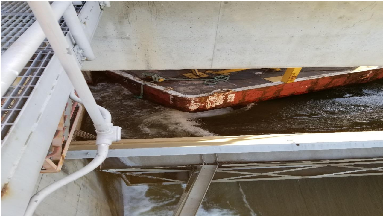
Appeared to be no contact with spill gate. Damage assessment continues.
